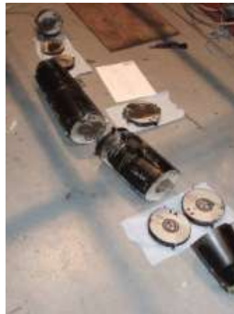
A 3 Core Heatshrink Joint incorporating a Shell and Resin design is cut in several places as part of the BS7888 test regime to check whether water has entered the joint.
